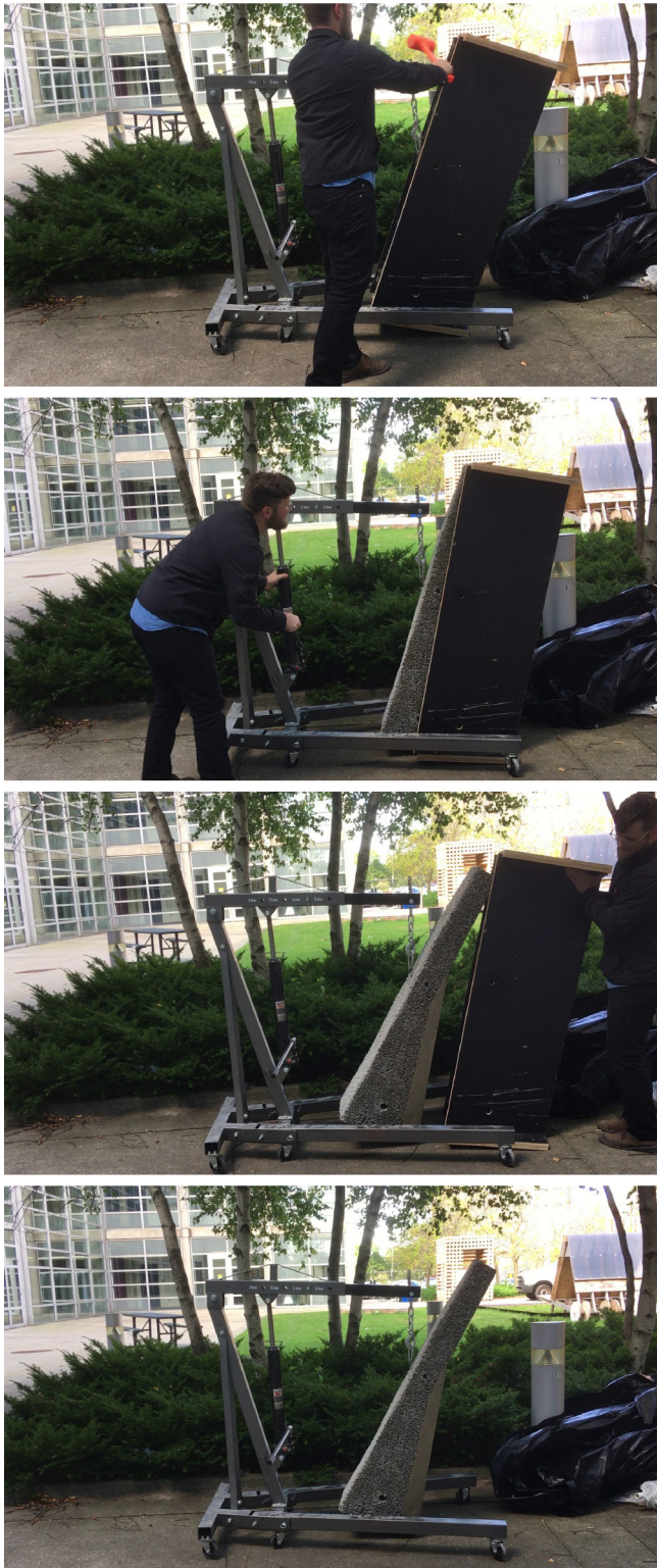
Figure 6. Pervious concrete must be wrapped in plastic to cure properly. Modules are moved with preset anchoring points. To remove the pieces an engine lift was used. Demolding was easy given the tapered form of the module.. Image Credit: Author
